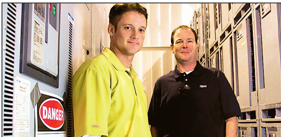
POWER PLAYERS: J.D. Dodson, left, and Brad Keating of Rapid Power Management review components at Jtek North America Inc's Ennis factory. For many companies, the cost of making their electric systems more efficient is recouped through lower electricity fees.
